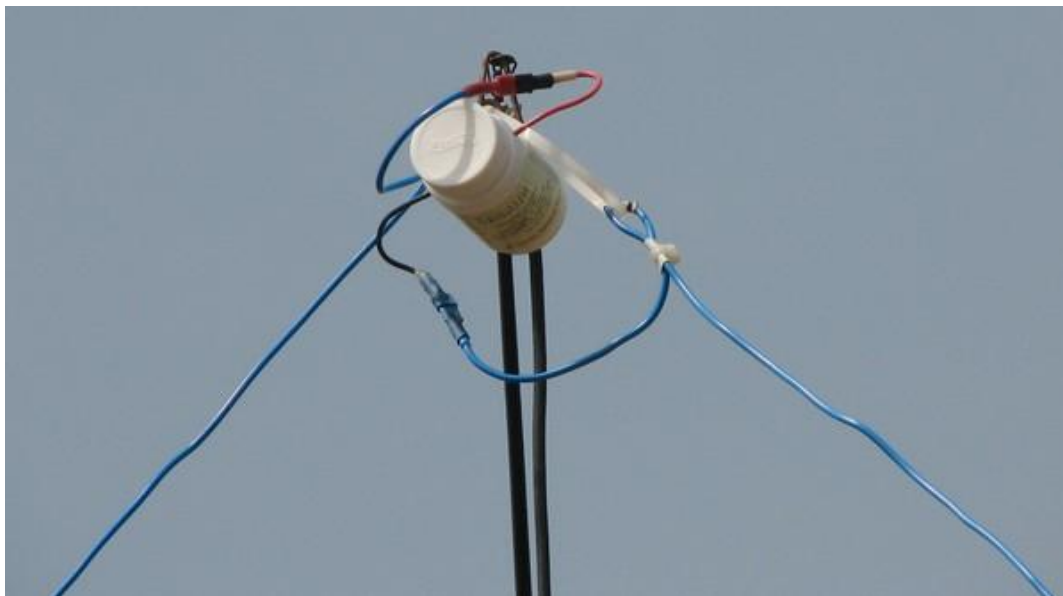
Matching Box on the Antenna
