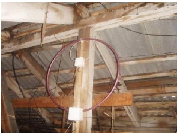
Picture 2 UA6AGW Antenna in the Attic
