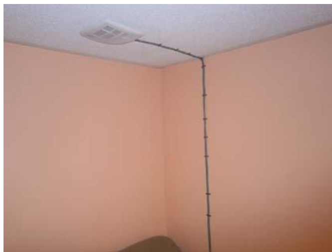
Picture 5 Coaxial Cable Going Into my Basement
