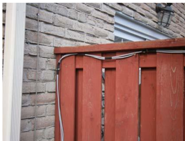
Picture 4 Coaxial Cable Going Along the Fence
